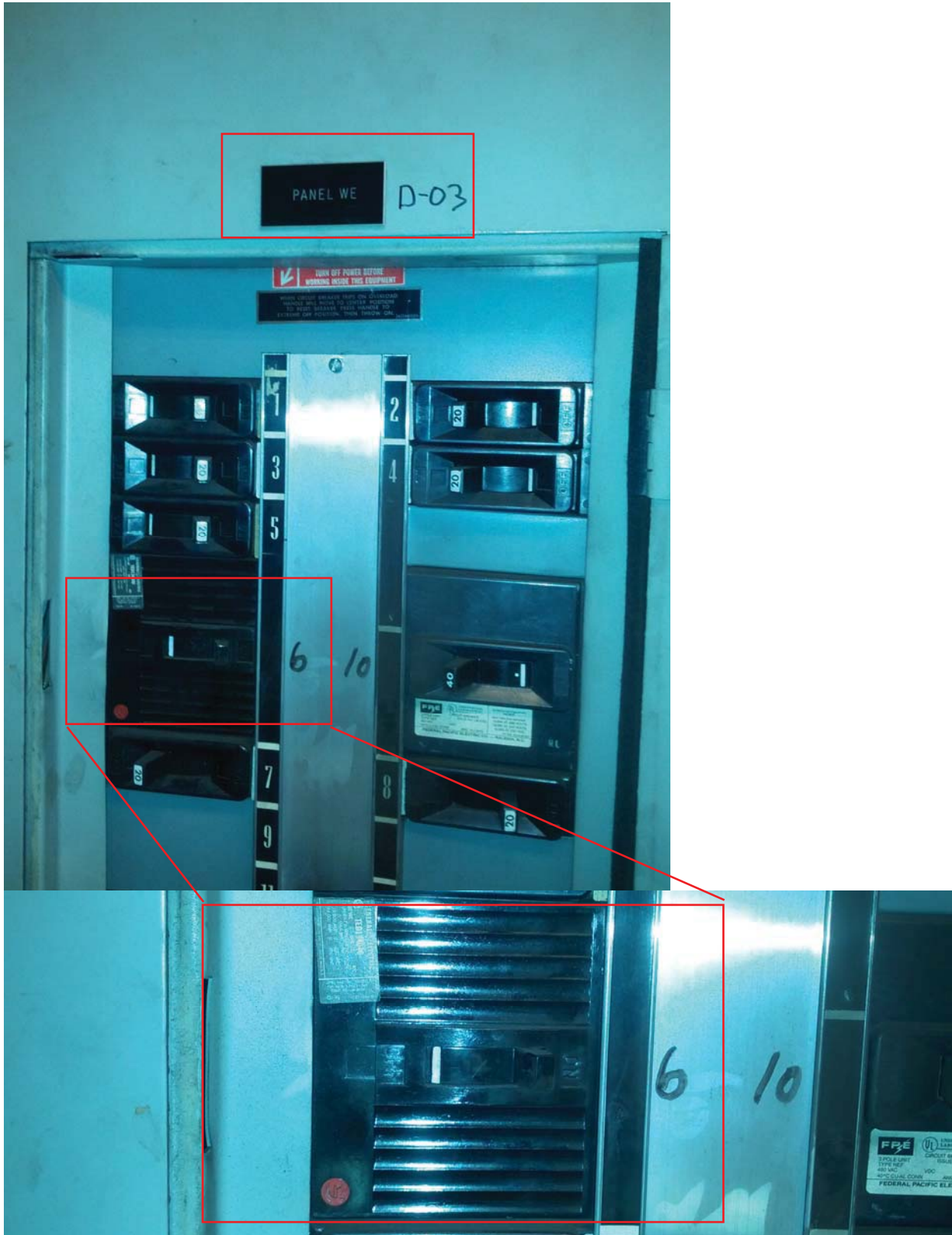
L'Enfant Plaza West Photo #5 – Source Panel (WE) for Panel WEZ which shares junction box with AFC Panel (WF) and has to be de-energized.
