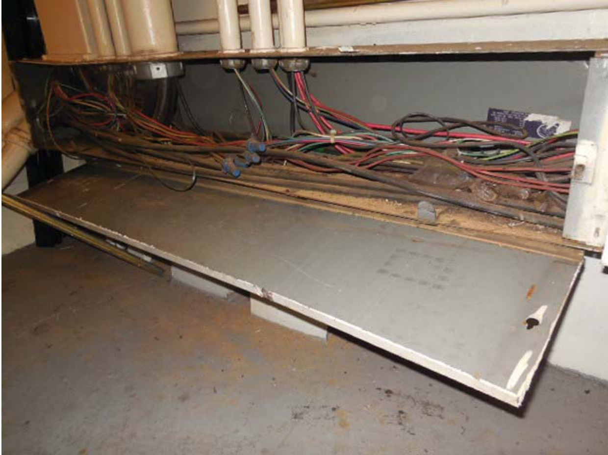
Picture 12: D02 Smithsonian North – Common trough for Panels NM, NM-E, NMH-E, NMH, & NMPO in Room 215
