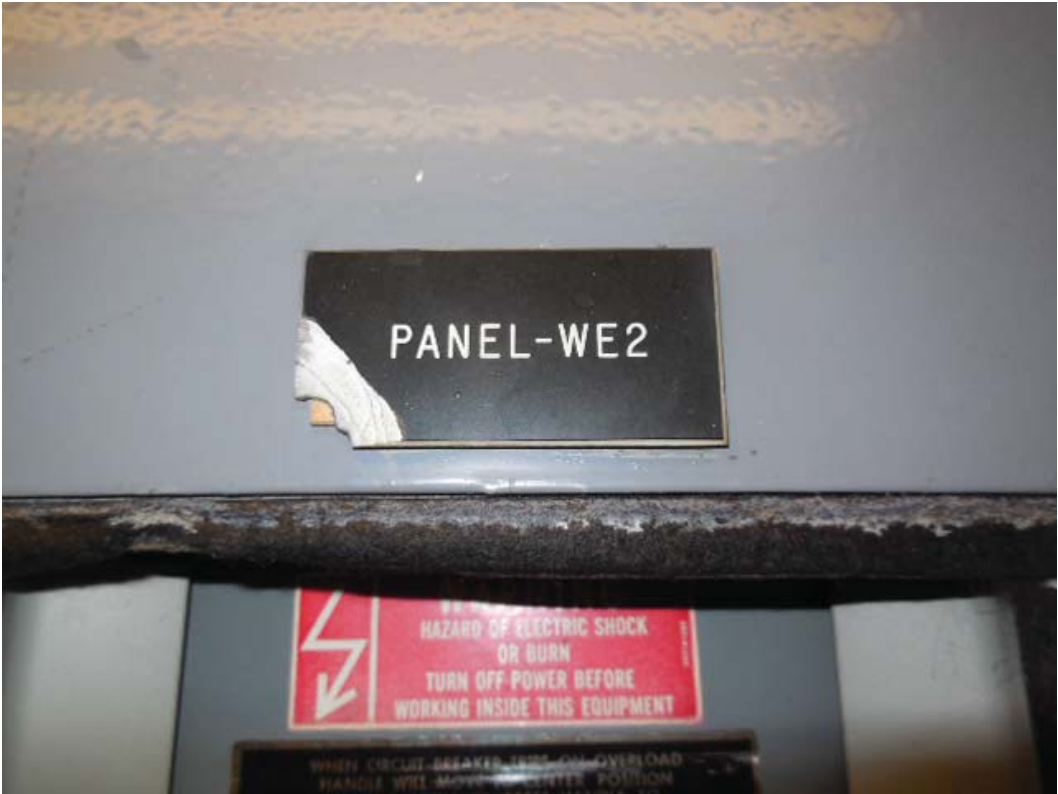
Picture 14: D01 Federal Triangle – Panel WE2 in room C206
