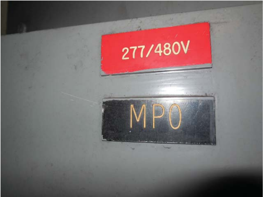
Picture 13: D05 Capitol South – Panel MPO in room C201
