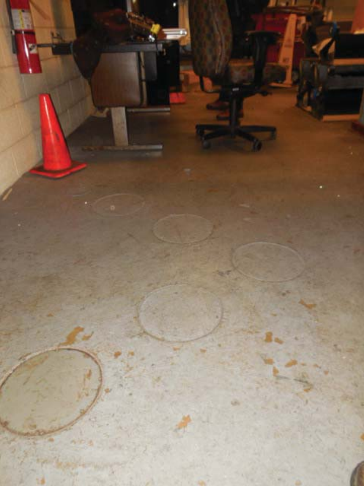
Picture 3: D02 Smithsonian North – Manholes in Service corridor
