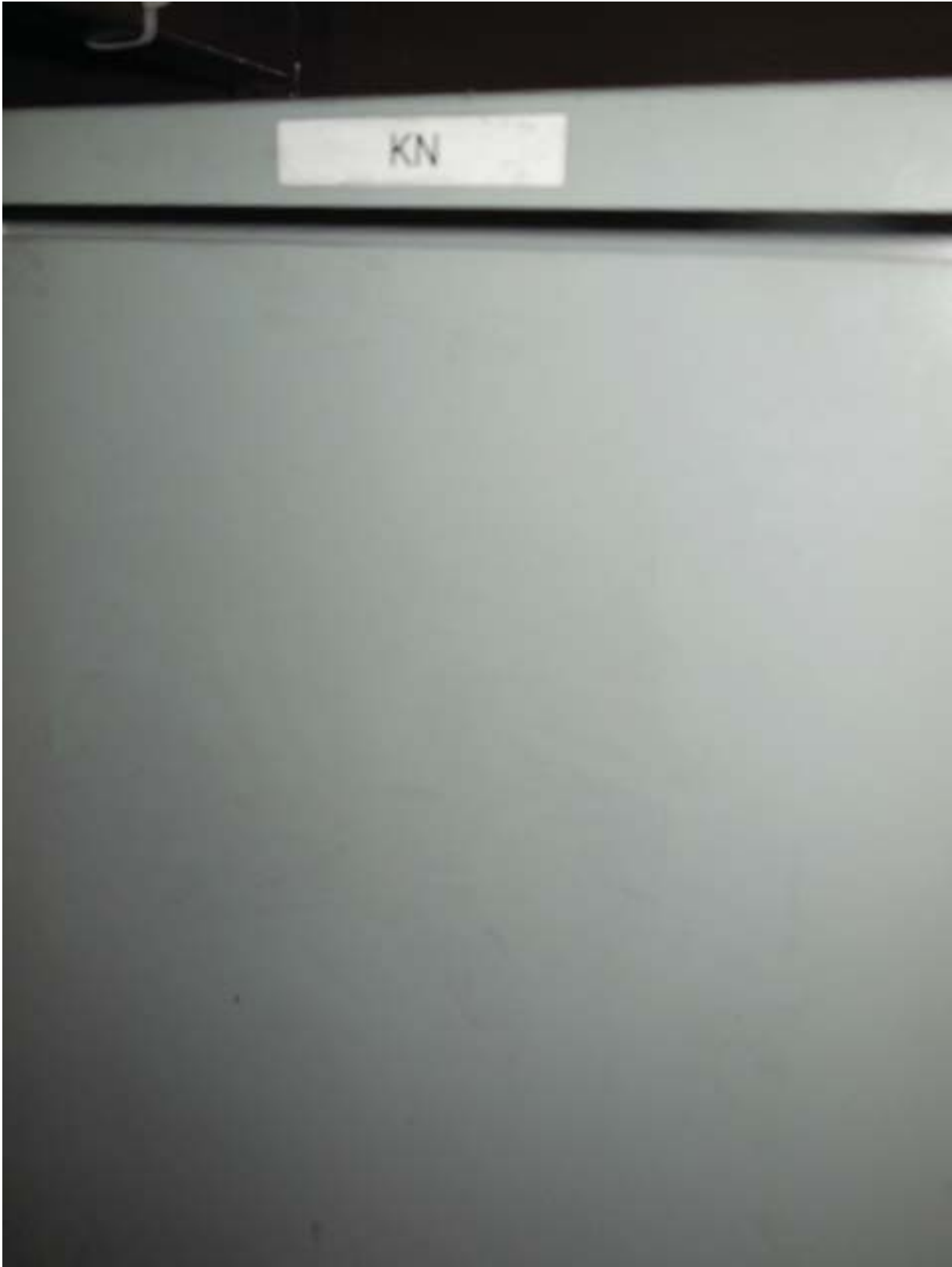
Picture 5: D02 Smithsonian South – Emergency Panel KN in Kiosk
