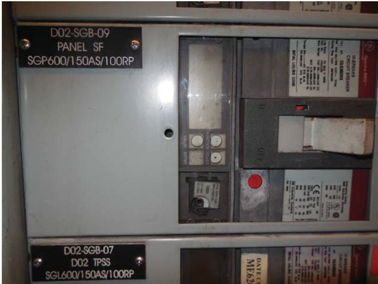
Picture 10: D02 Smithsonian South – Breaker D02-SGB-09 for Panel SF in Room 104
