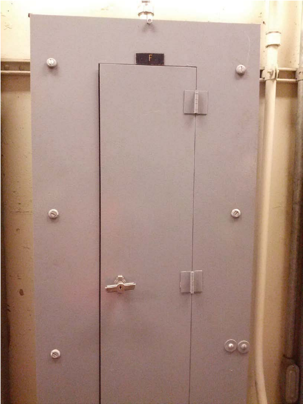
Picture 8: D04 Federal Center SW – AFC Panel F in room 206
