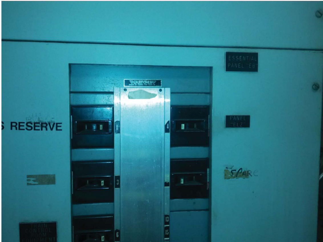
L'Enfant Plaza East Photo #4 –AFC Source Switchboard (EB) located in Room #103 on Platform Level Track 1 Wayside. Source Breaker (Panel “EF”) Circuit #7 for AFC Panel (EB).
