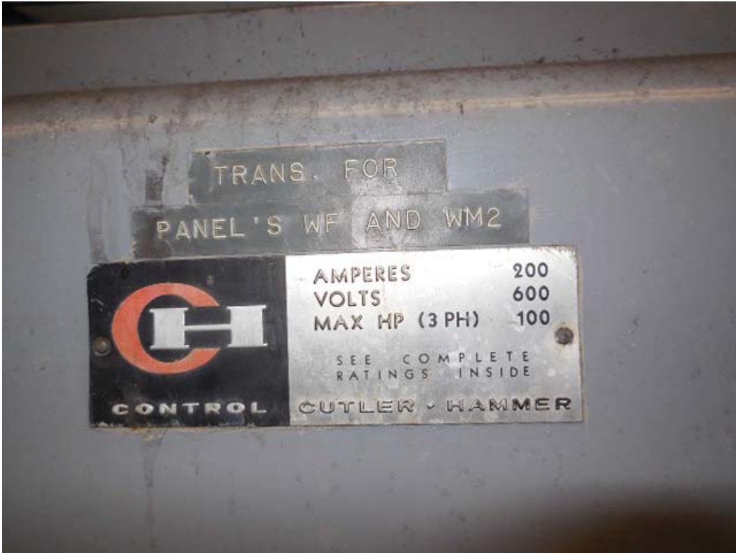
Picture 13: D01 Federal Triangle – Transformer for Panels WF and WM2 in room C206
