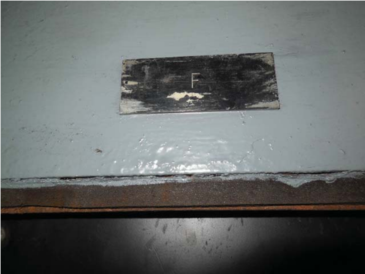
Picture 6: D06 Eastern Market – AFC Panel F in Room C206
