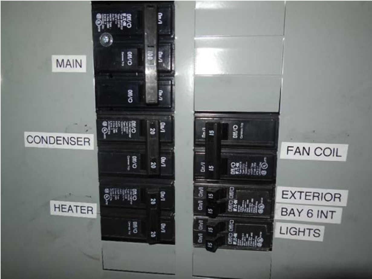
Picture 6: D02 Smithsonian North – Unknown Emergency Panel in Kiosk
