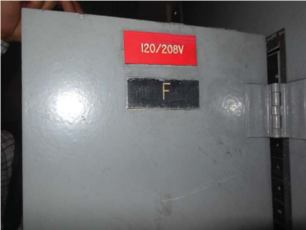
Picture 9: D05 Capitol South – AFC Panel F in room C201
