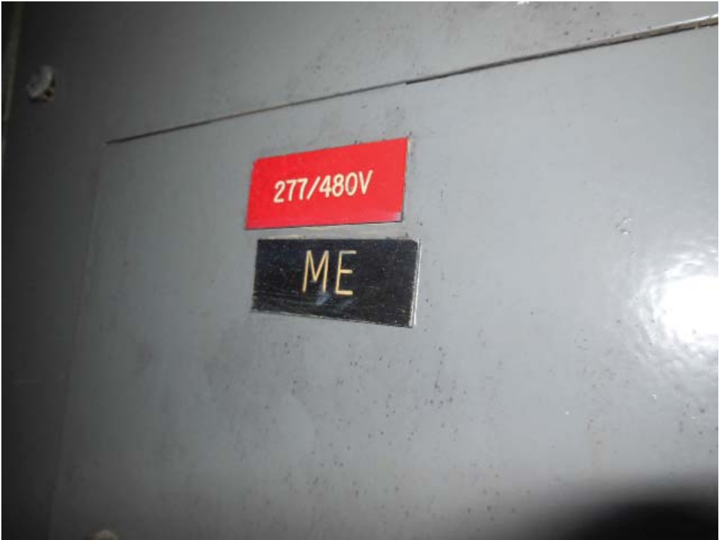
Picture 12: D05 Capitol South – Panel ME in room C201
