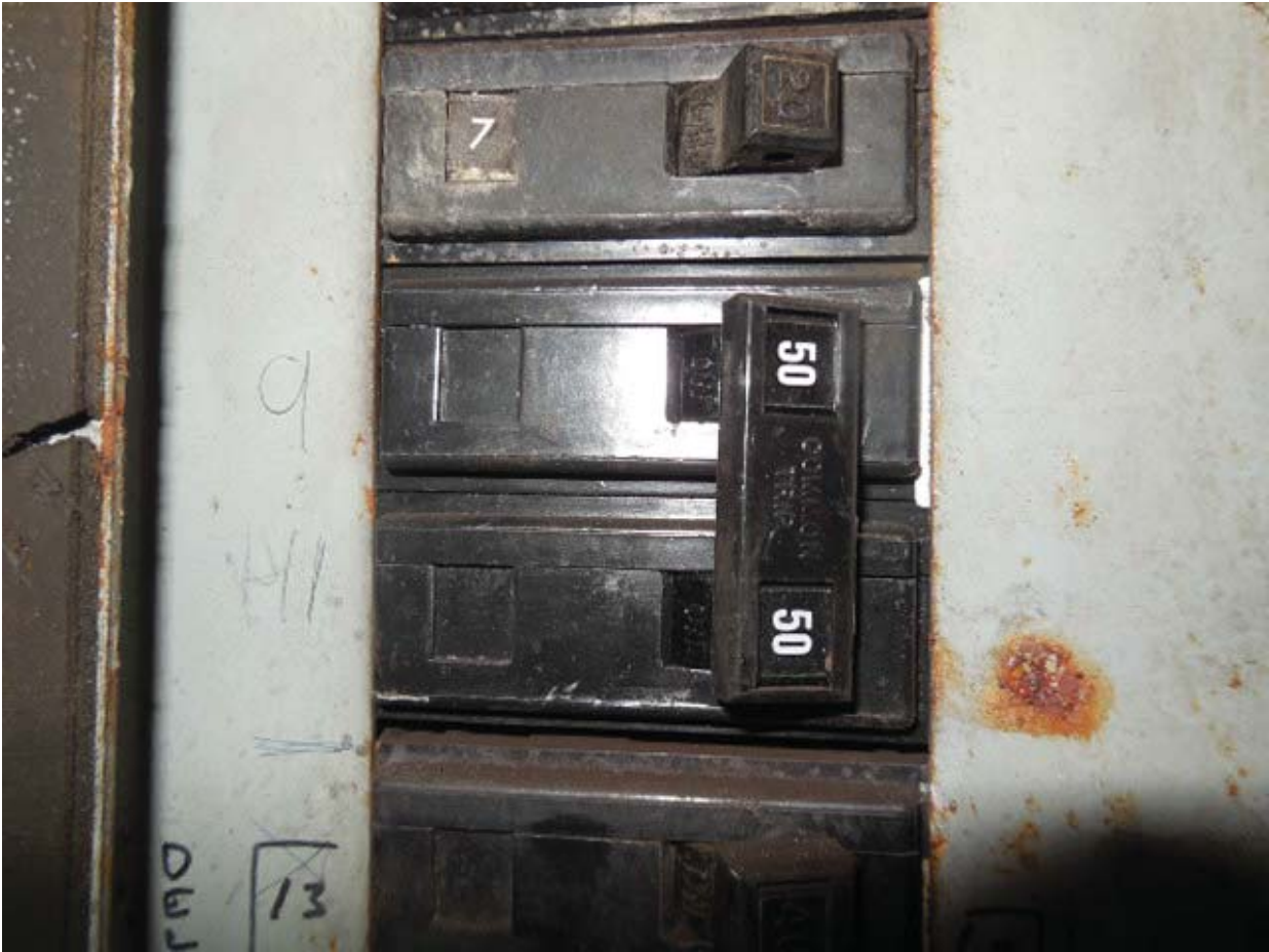
Picture 13: D06 Eastern Market – Panel MEP in Room C206 – Circuits 9 & 11
