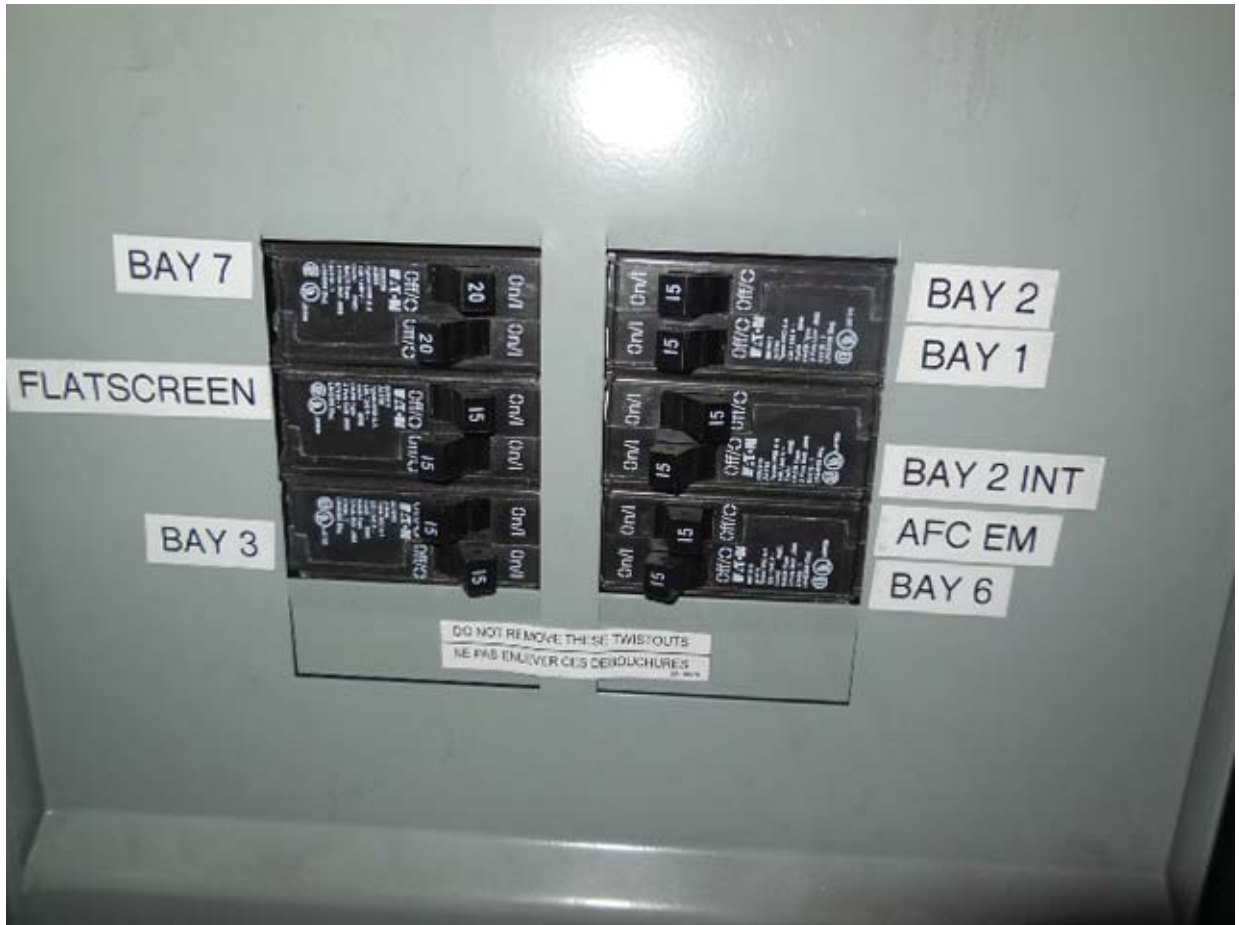
Picture 5: D02 Smithsonian North – Emergency Panel KE in Kiosk
