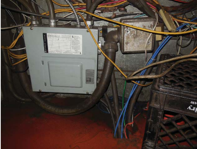
Pictures 5&6: D01 Federal Triangle – Emergency panel in Kiosk
