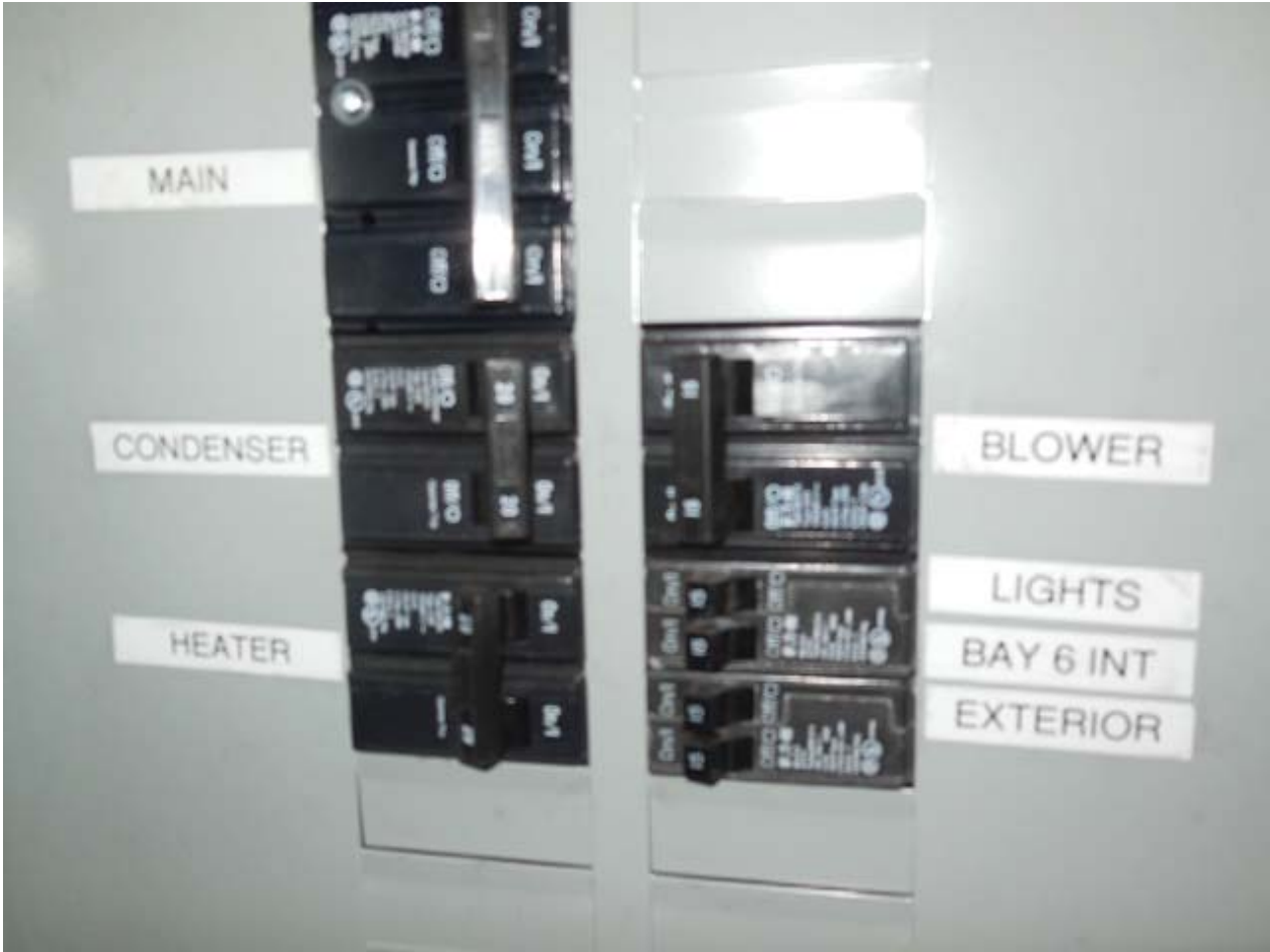
Picture 4: D02 Smithsonian South – Emergency Panel KE in Kiosk
