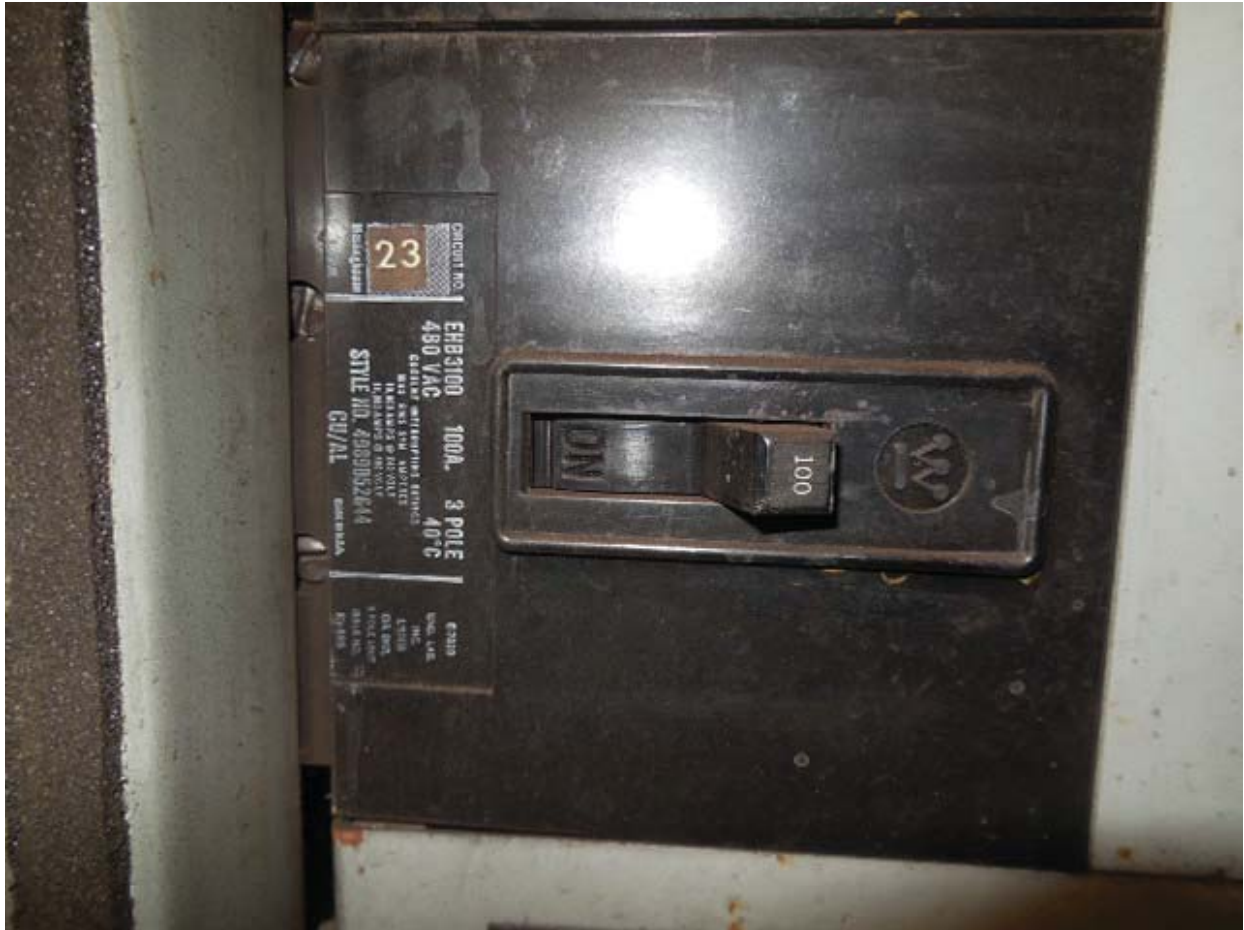
Picture 10: D06 Eastern Market – Panel MPB in Room C206
