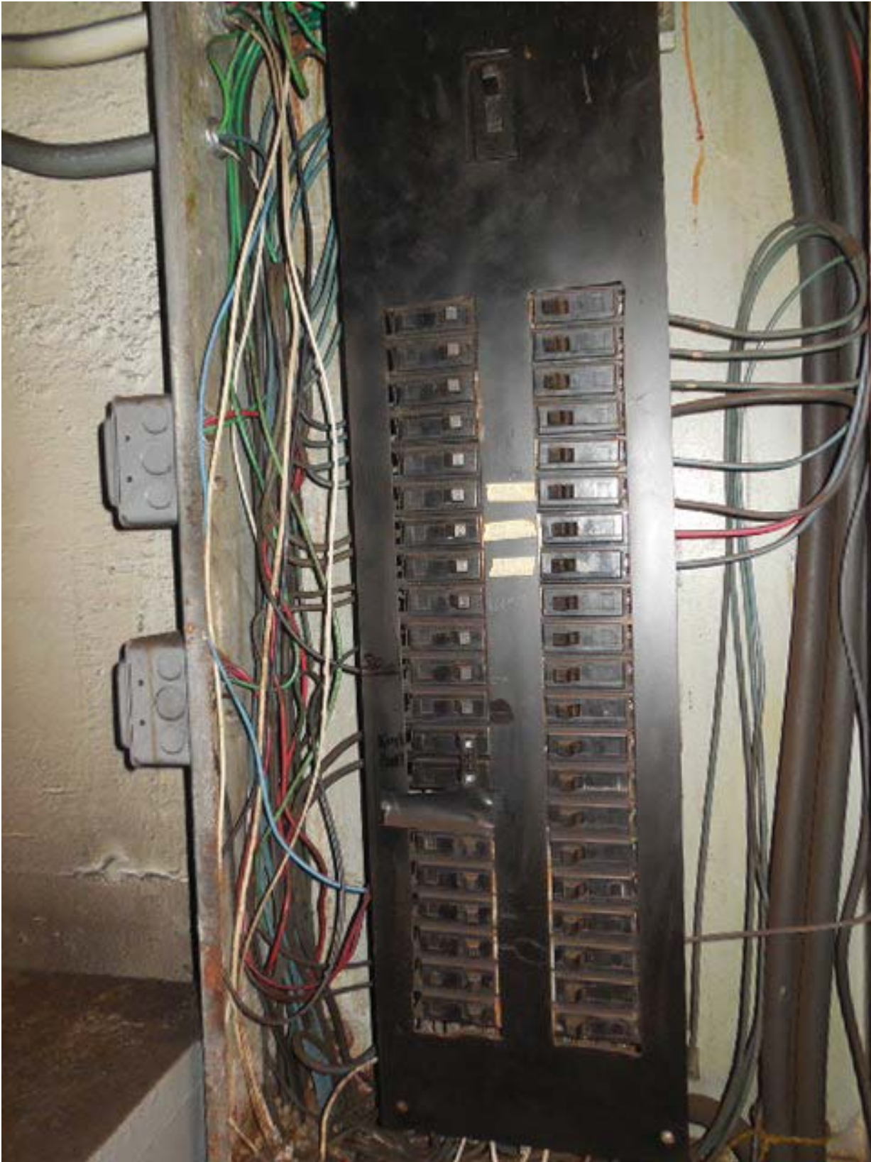
Picture 7: D06 Eastern Market – AFC Panel F in Room C206
