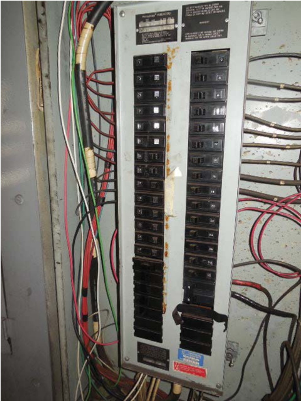
Picture 10: D05 Capitol South – AFC Panel F in room C201
