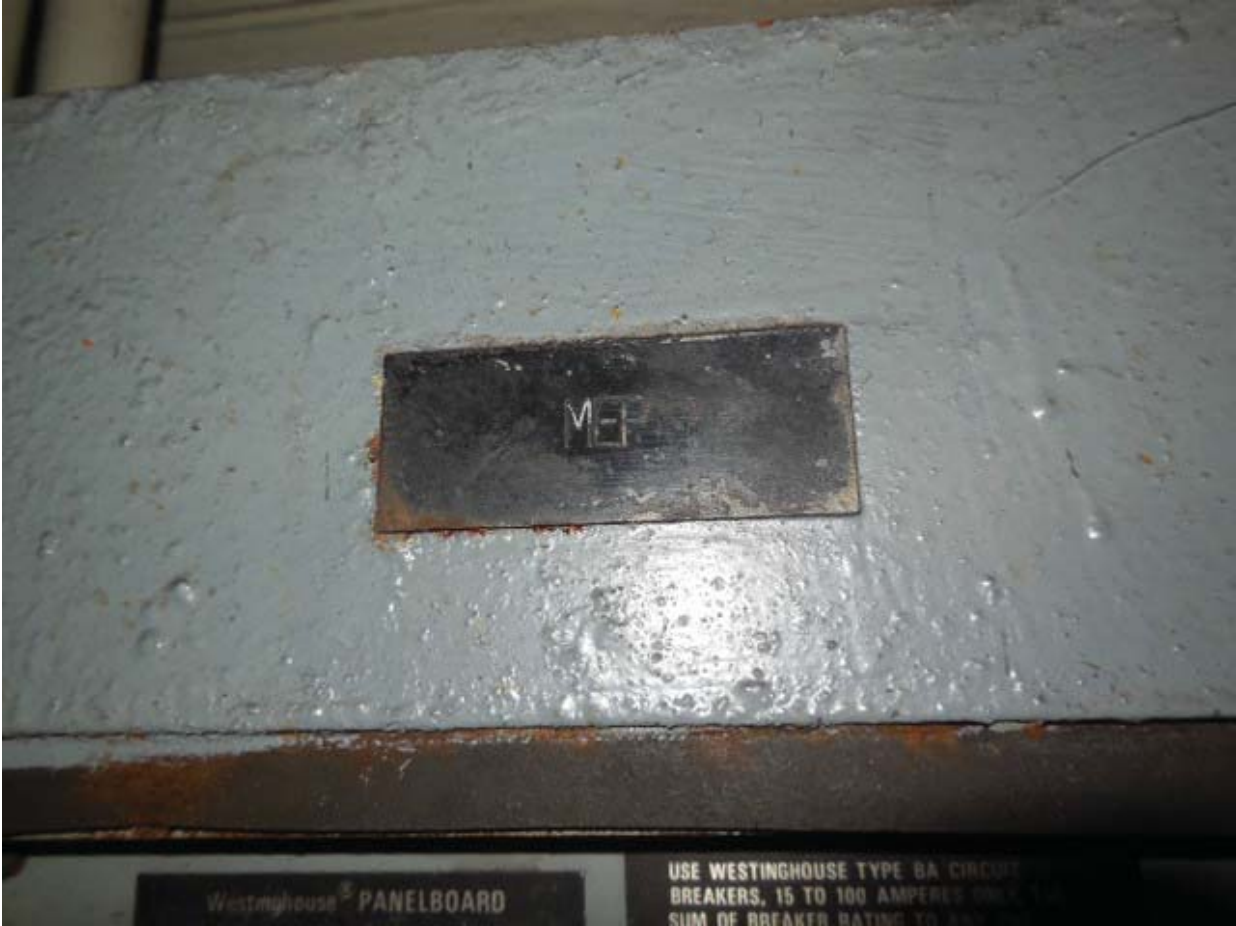
Picture 12: D06 Eastern Market – Panel MEP in Room C206
