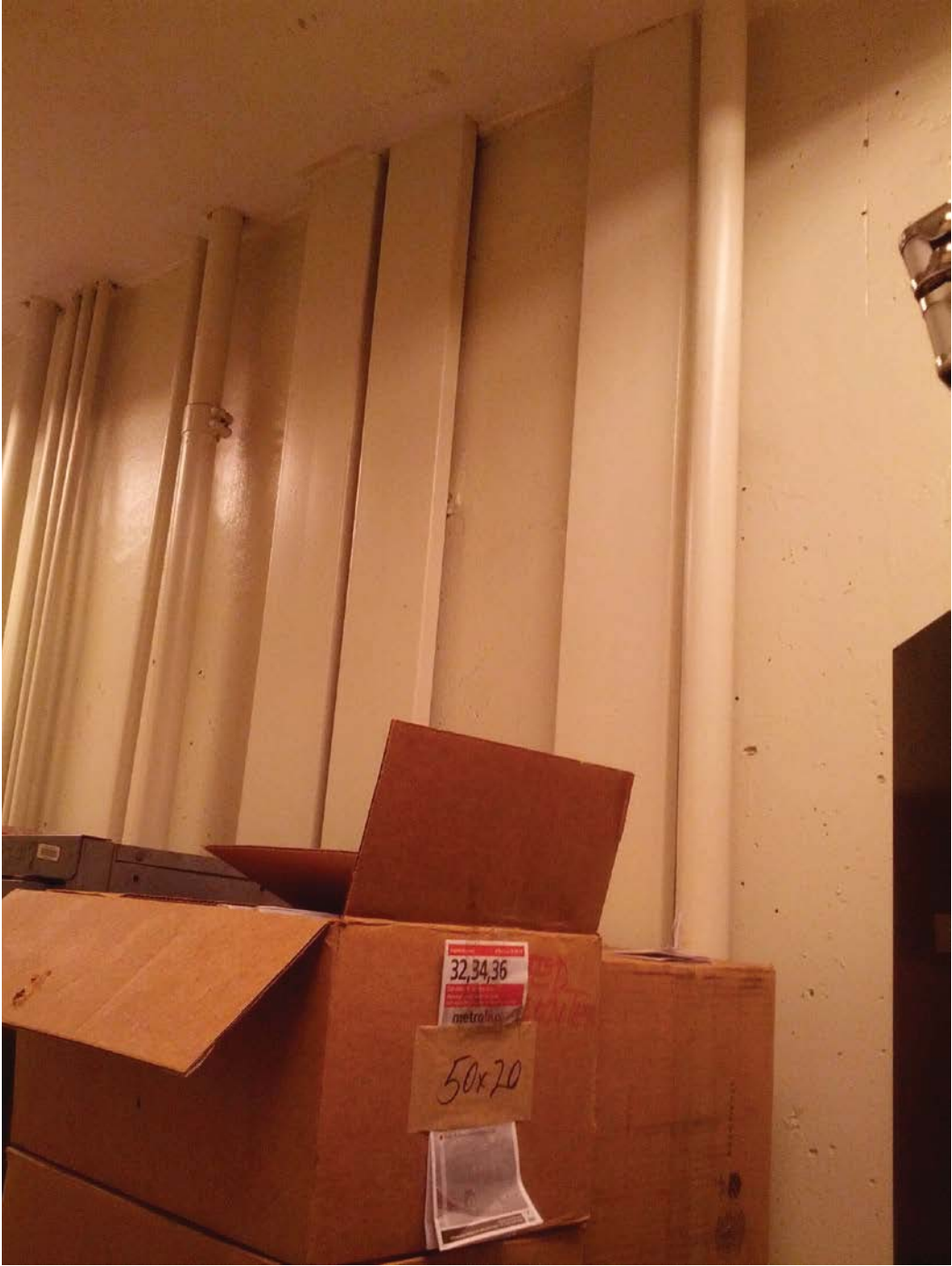
Picture 5: D04 Federal Center SW – Ducts & conduits running up wall in maintenance corridor
