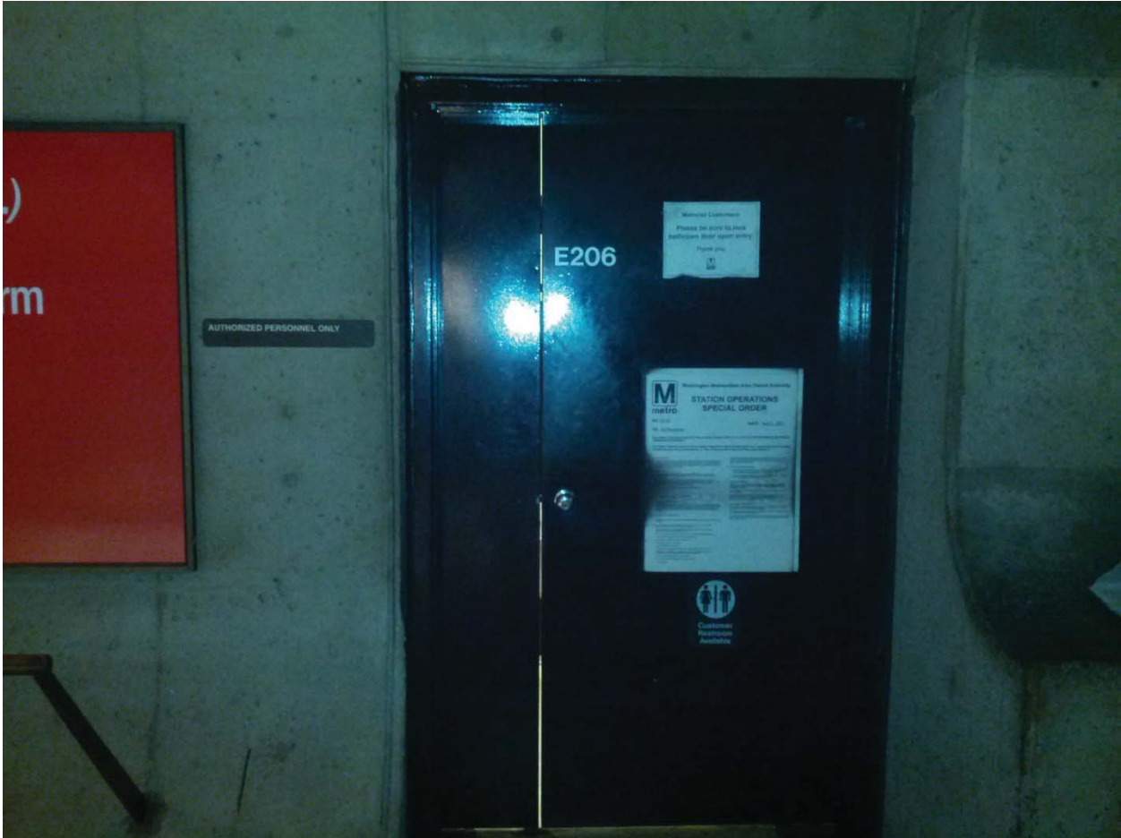
L'Enfant Plaza East Photo #5 – AFC Panel (EF) - Room E206 (Mezzanine Level)
