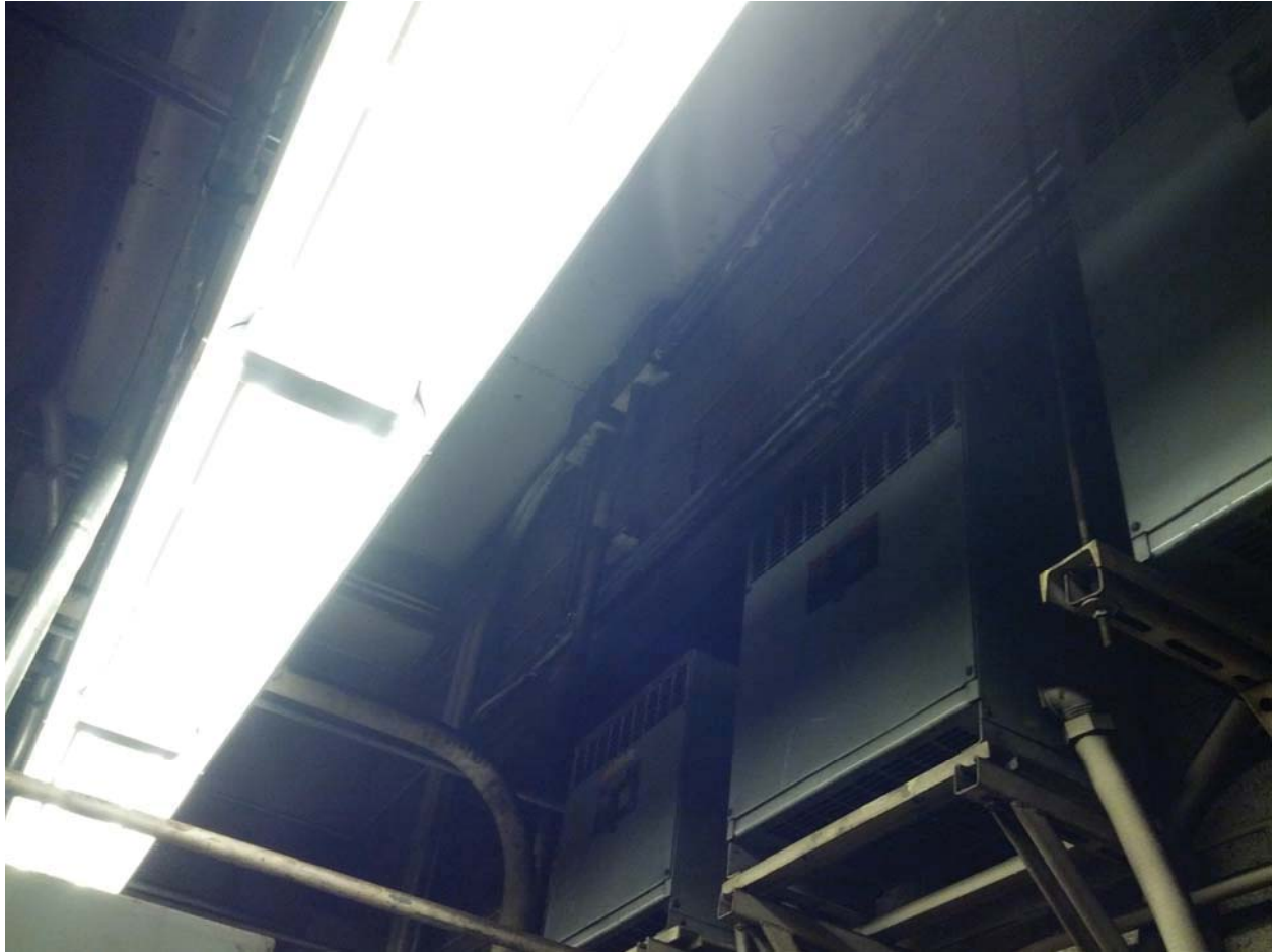
L'Enfant Plaza West Photo #7 –Shared Junction Box for AFC Panel (WF) and Panel (WEZ) where overhead conduits land in same junction box. Platform Level in Rm. W104 Track 1 Wayside.
