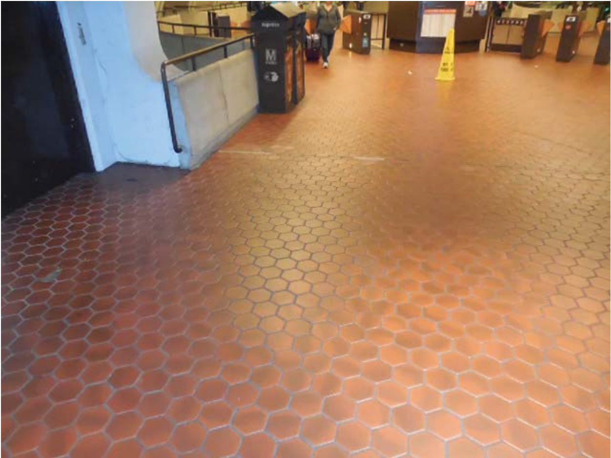
Picture 1: D02 Smithsonian South – No handholes on Mezzanine
