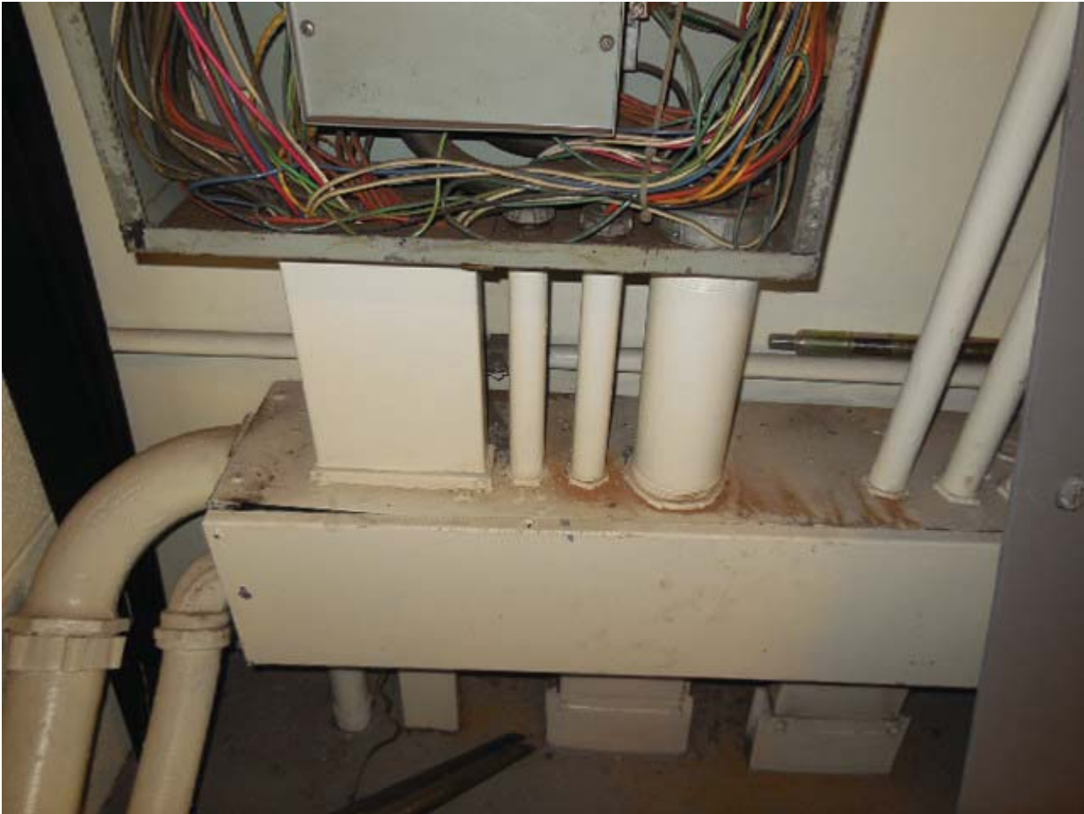
Picture 10: D02 Smithsonian North – AFC Panel NF in Room 215 – Bottom duct & conduits
