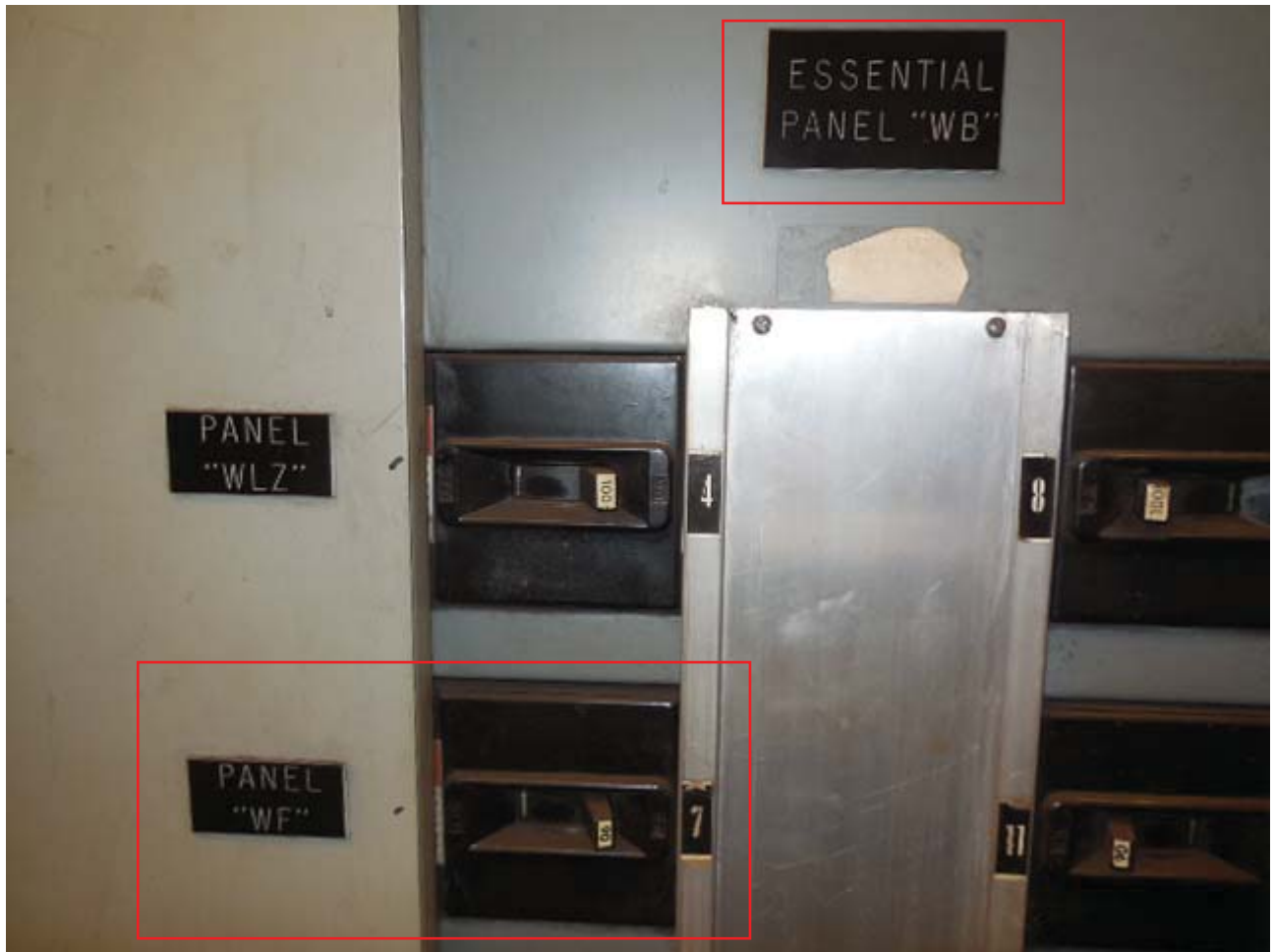
L'Enfant Plaza West Photo #4 - AFC Source Switchboard (WB) located in Room #W104 on Platform Level Track 1 Wayside. Source Breaker (Panel "WF") Circuit #7 for AFC Panel (WF).
