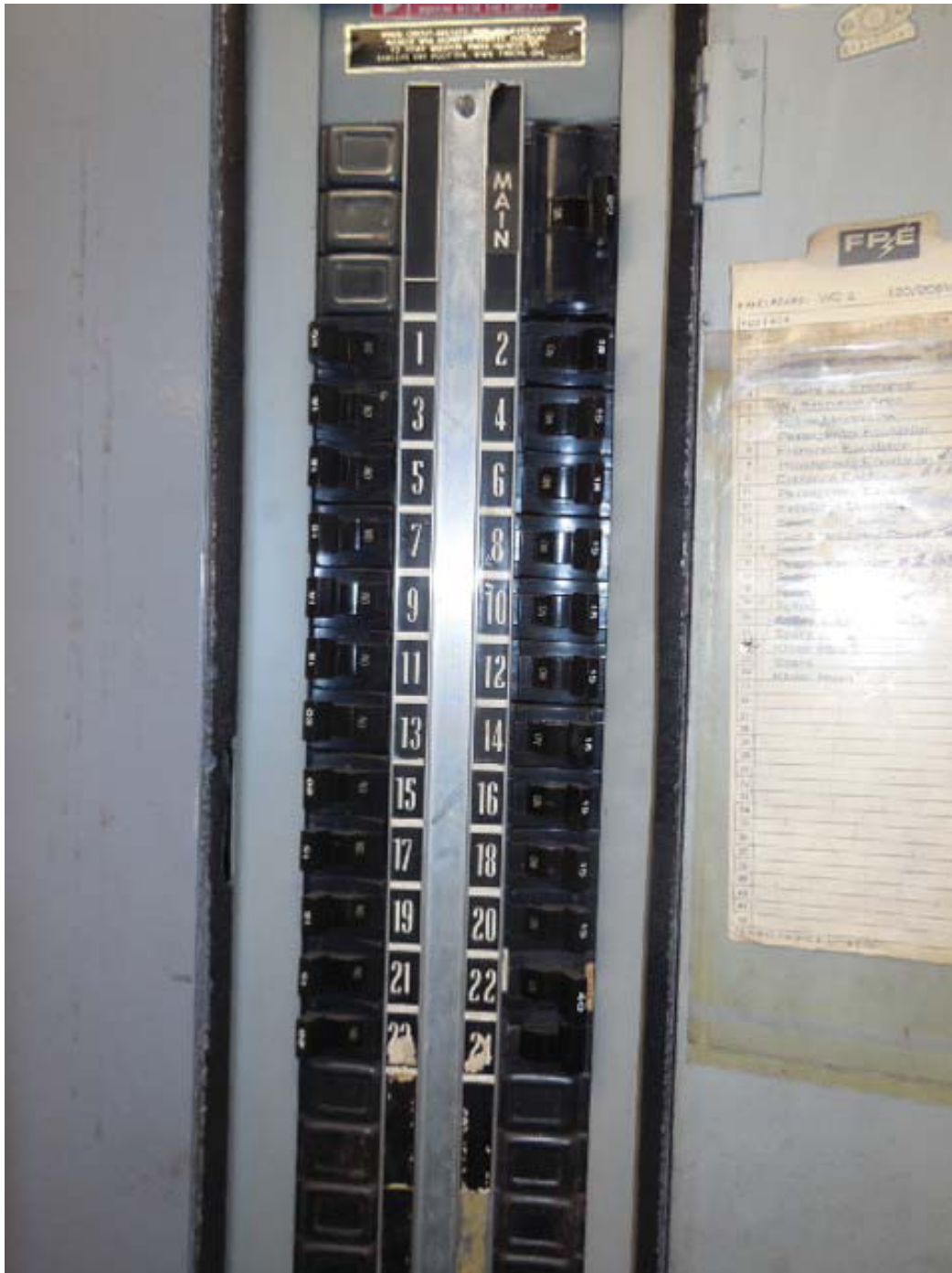
Picture 15: D01 Federal Triangle – Panel WE2 in room C206
