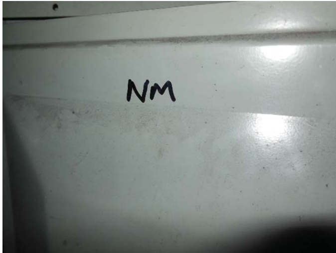
Pictures 6-8: D05 Capitol South – Emergency panel NM in Kiosk
