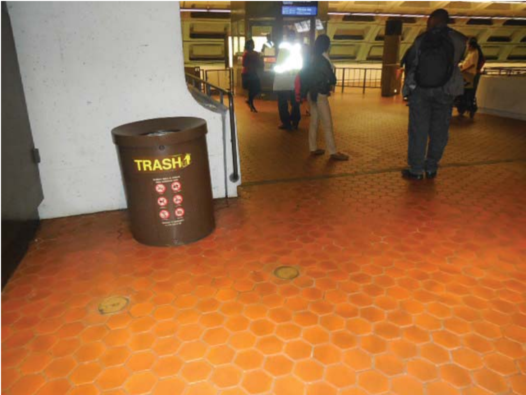
Pictures 1&2: D04 Federal Center SW – Handholes and manhole in mezzanine
