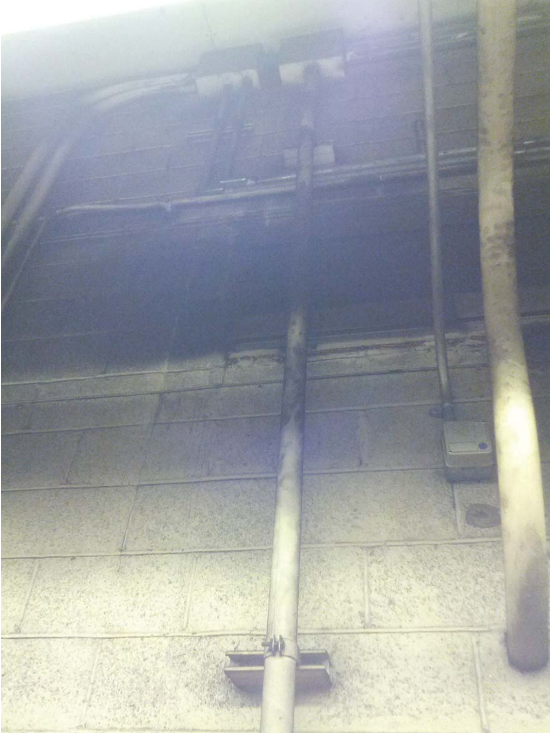
L'Enfant Plaza West Photo #8 –Shared Junction Box for AFC Panel (WF) and Panel (WEZ) where overhead conduits land in same junction box. Platform Level in Rm. W104 Track 1 Wayside.
