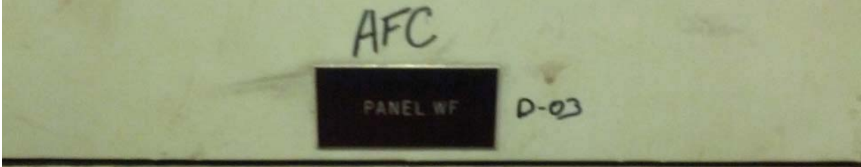
L'Enfant Plaza West Photo #1 – AFC Panel (WF) Located on Platform Level Track 1 Wayside (Rm. W104)
