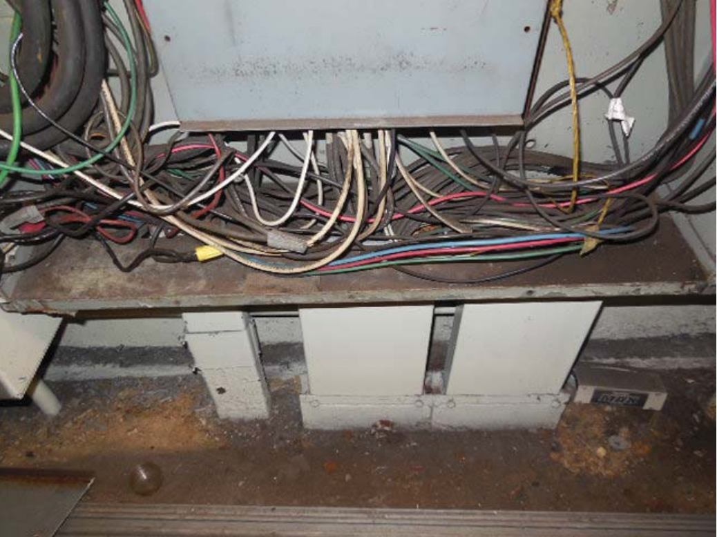
Picture 9: D01 Federal Triangle – AFC Panel WF in room C206 – Bottom ducts and conduit
