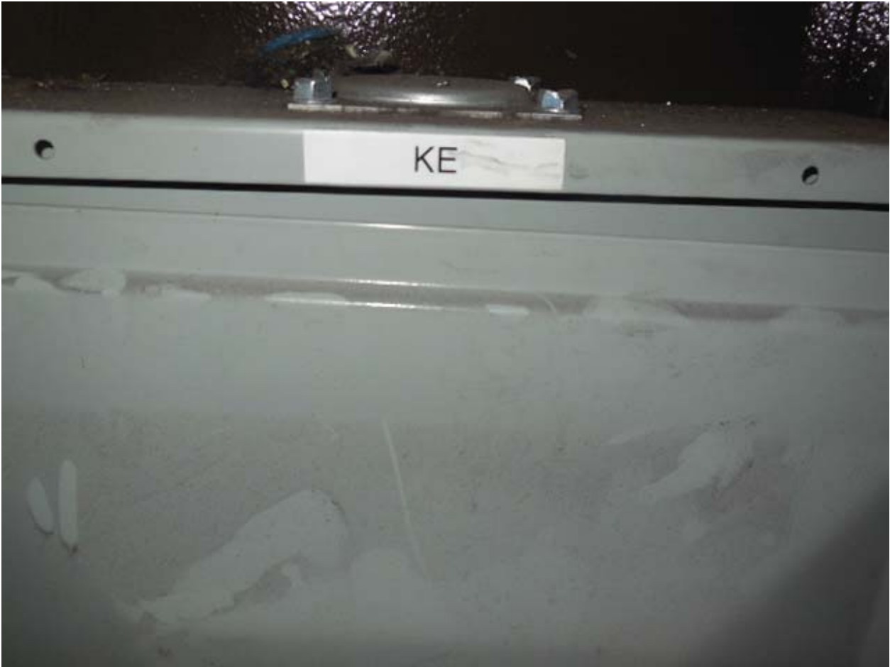
Picture 2: D02 Smithsonian South – Emergency Panel KE in Kiosk
