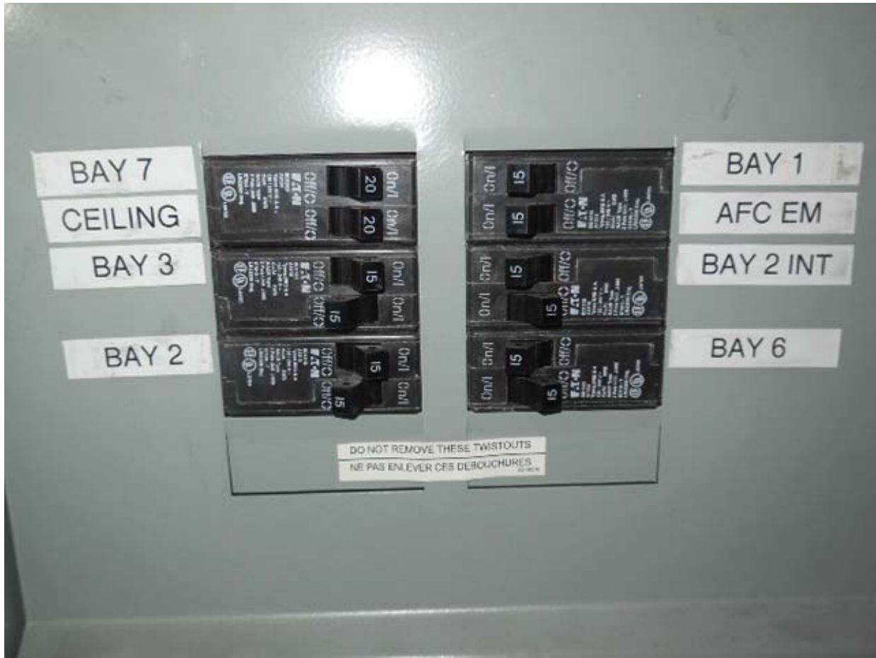
Picture 3: D02 Smithsonian South – Emergency Panel KE in Kiosk
