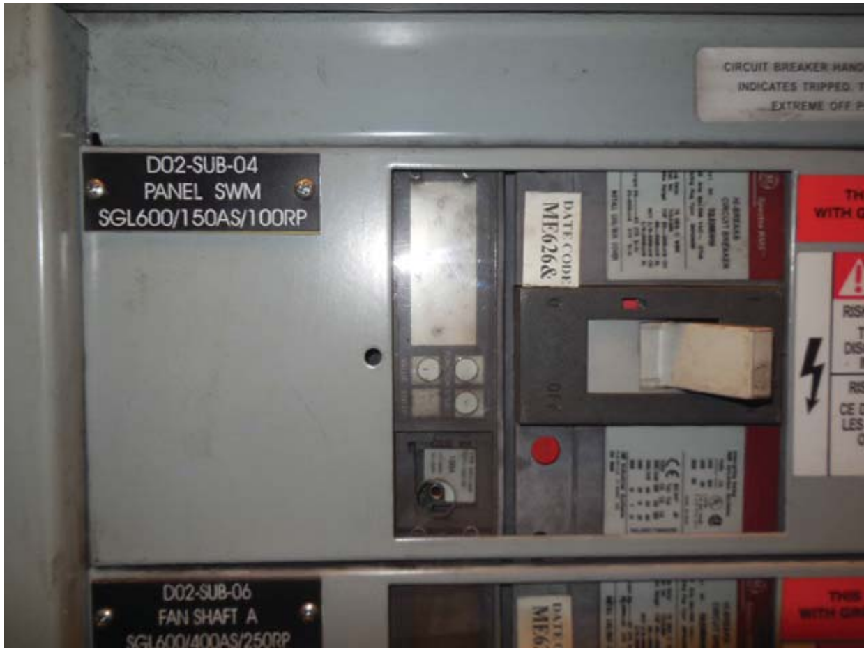
Picture 11: D02 Smithsonian South – Breaker D02-SUB-04 for Panel SWM in Room 104
