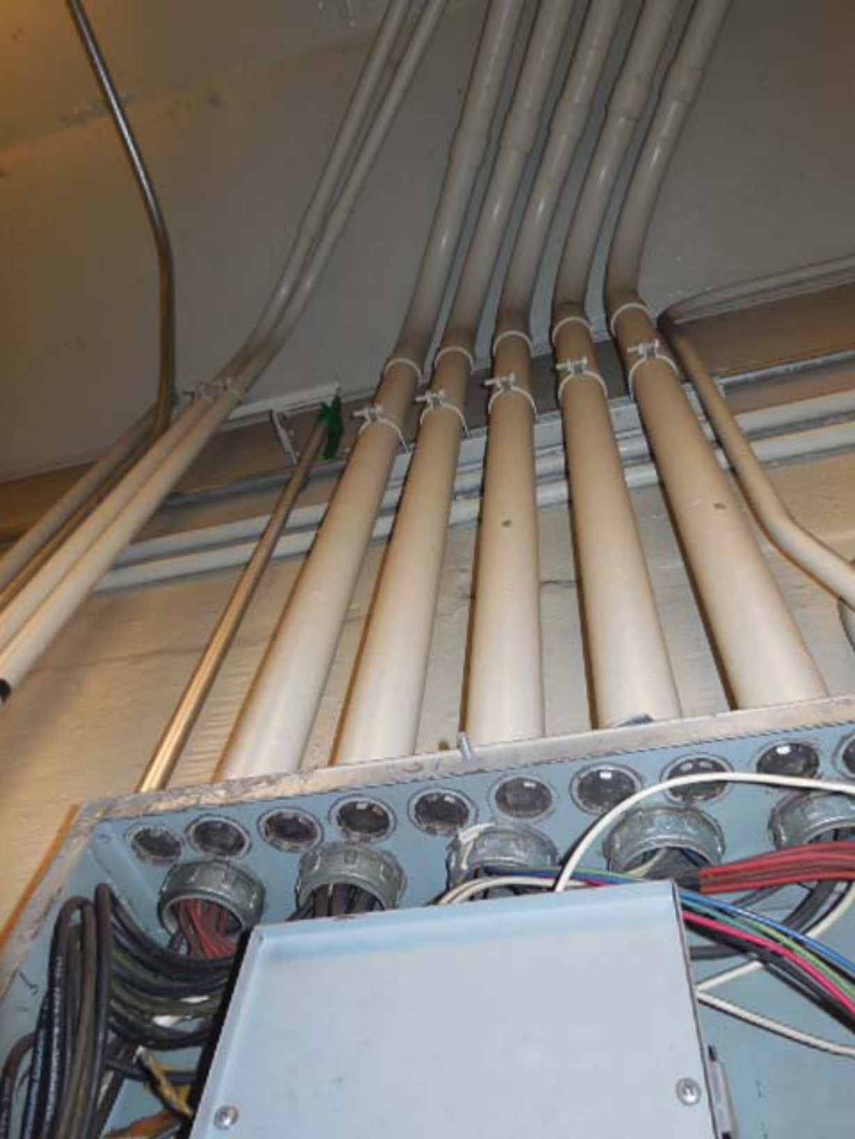
Picture 9: D02 Smithsonian South – AFC Panel SF in Room 104 – Conduits above panel
