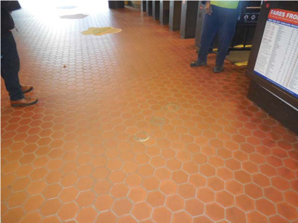
Picture 2: D02 Smithsonian North – Handholes on Mezzanine
