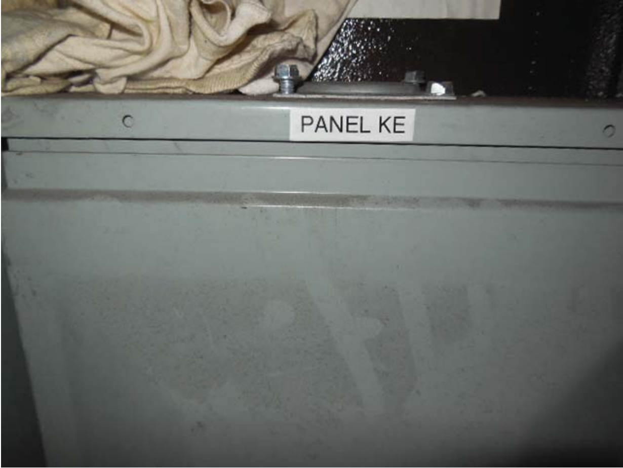
Picture 4: D02 Smithsonian North – Emergency Panel KE in Kiosk
