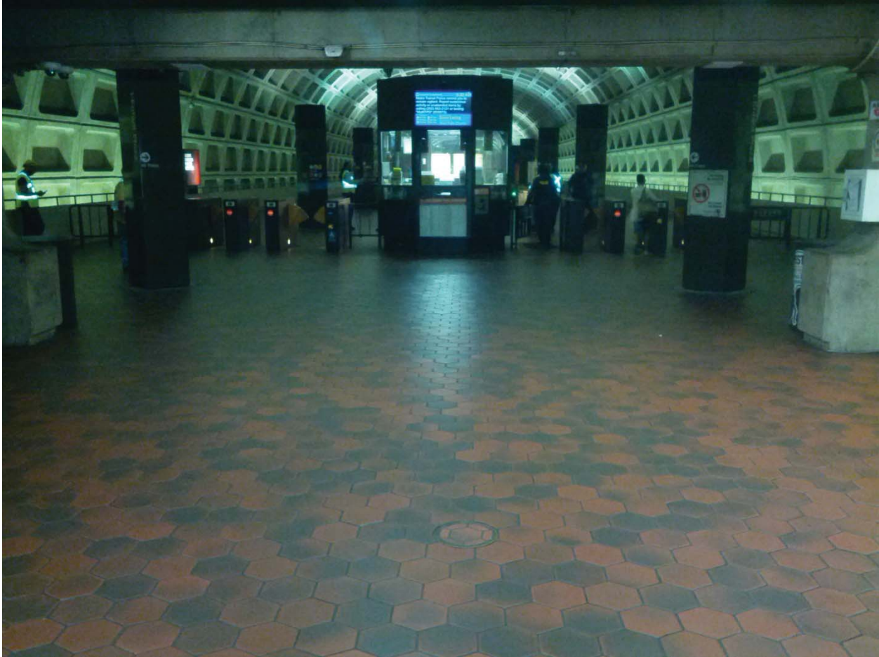
L'Enfant Plaza North Photo #11 – Handhole located on Mezzanine Level about 40' from Kiosk
