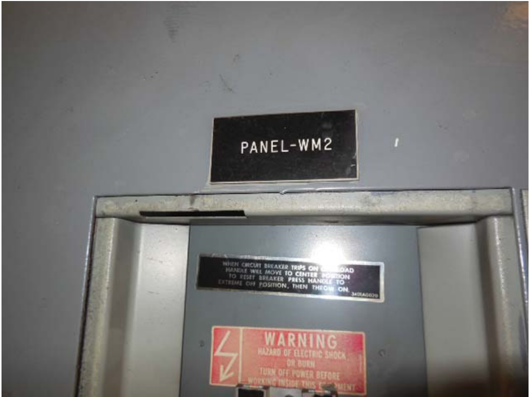
Picture 11: D01 Federal Triangle –Panel WM2 in room C206
