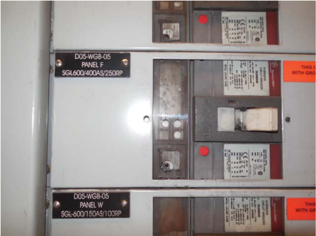
Picture 16: D05 Capitol South – SWBD circuit for D05-WGB-05 Panel F in room 309
