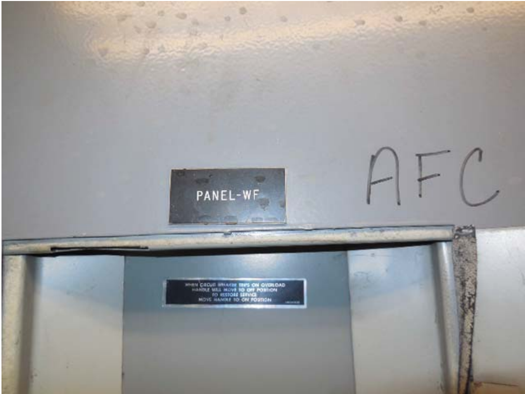
Picture 7: D01 Federal Triangle – AFC Panel WF in room C206
