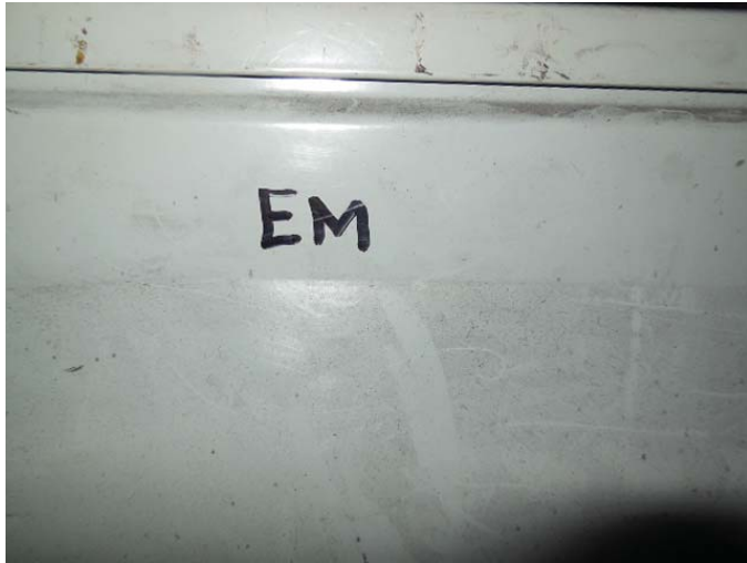
Pictures 3-5: D05 Capitol South – Emergency panel EM in Kiosk
