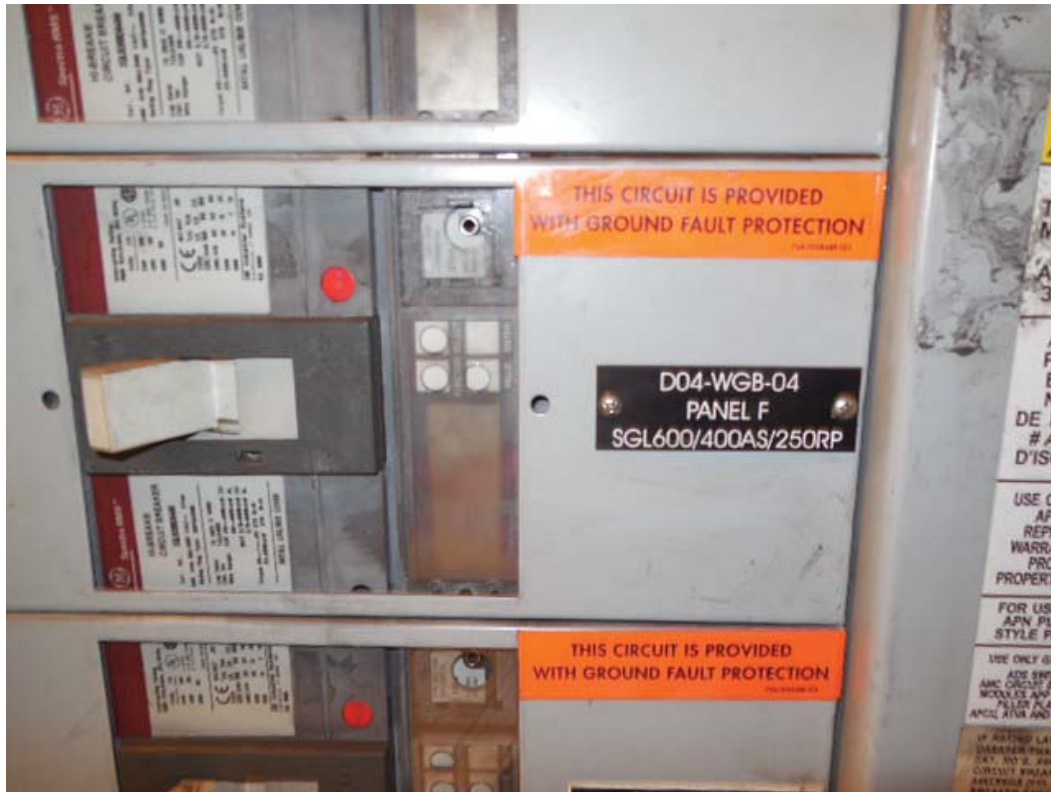
Picture 11: D04 Federal Center SW – SWBD circuit D04-WGB-04 Panel F in room C203
