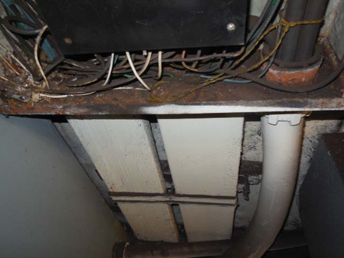
Picture 8: D06 Eastern Market – AFC Panel F in Room C206 – Ducts below Panel
