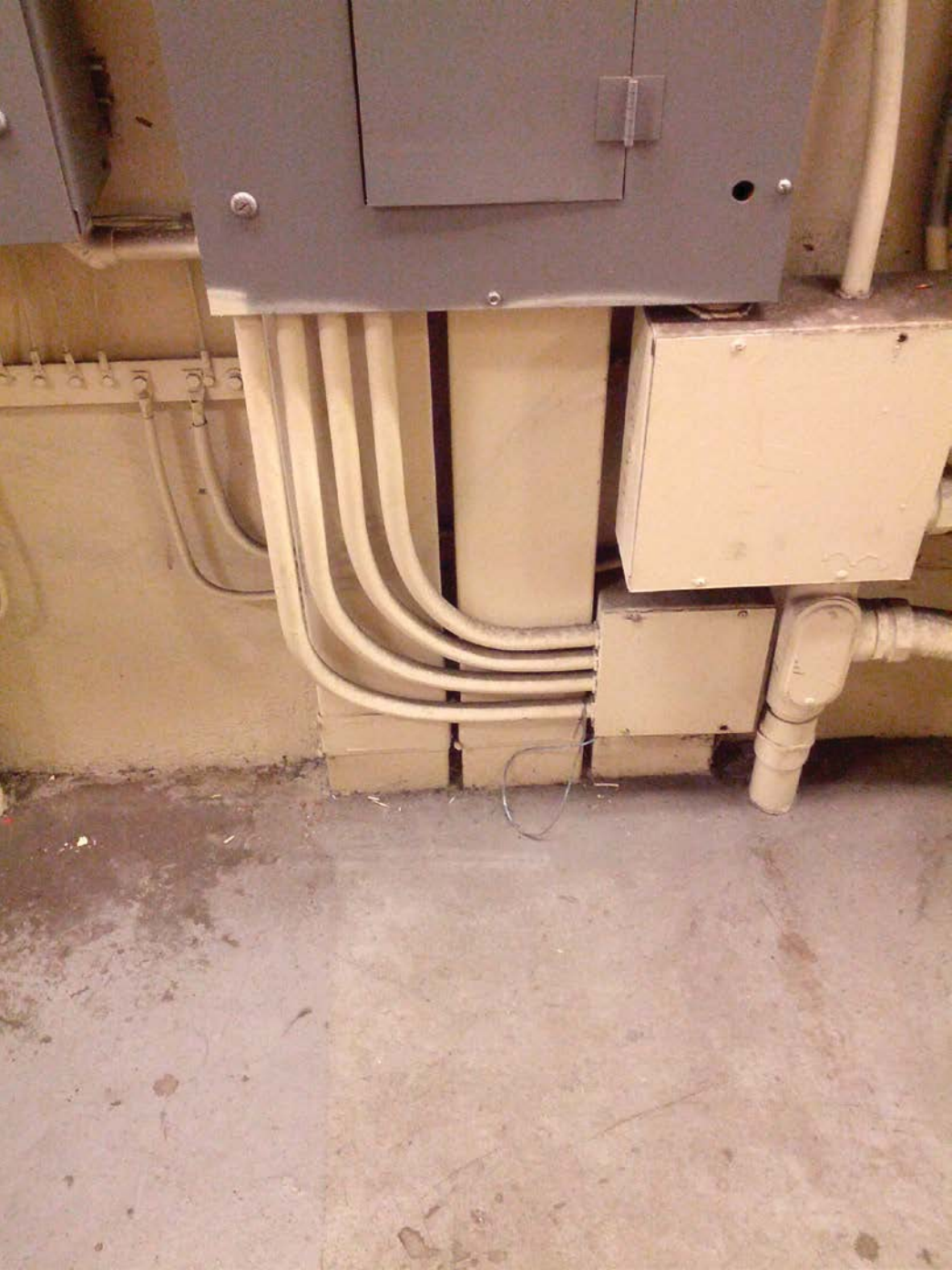
Picture 9: D04 Federal Center SW – AFC Panel F in room 206, Bottom ducts & conduits
